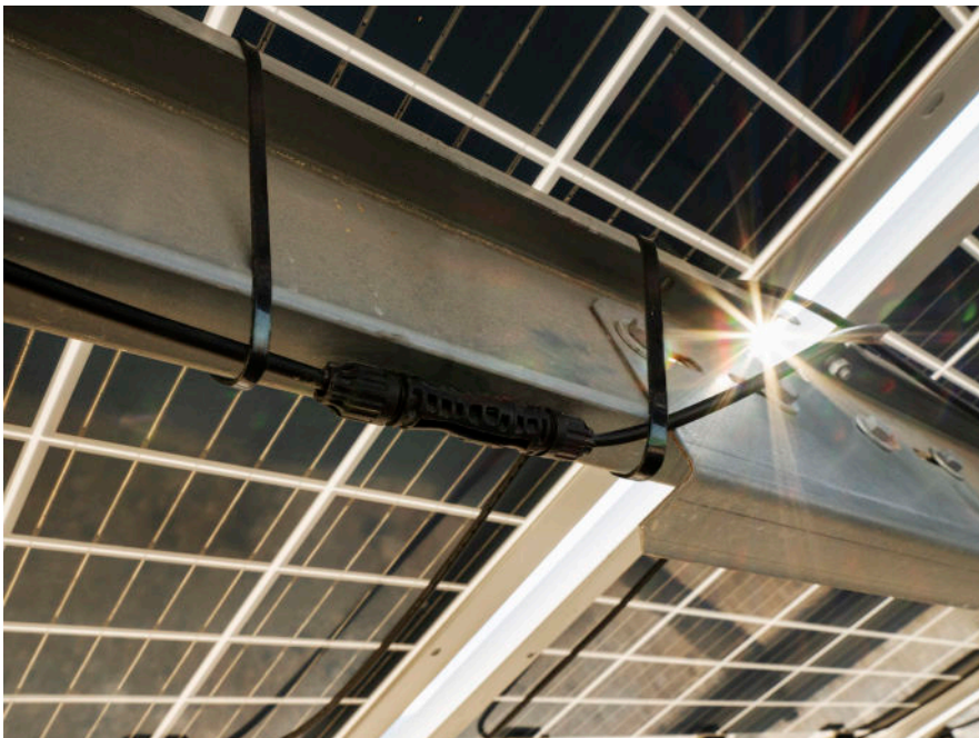
The DC wiring system with cable couplers, or eBOS, is the lifeline of a PV system
