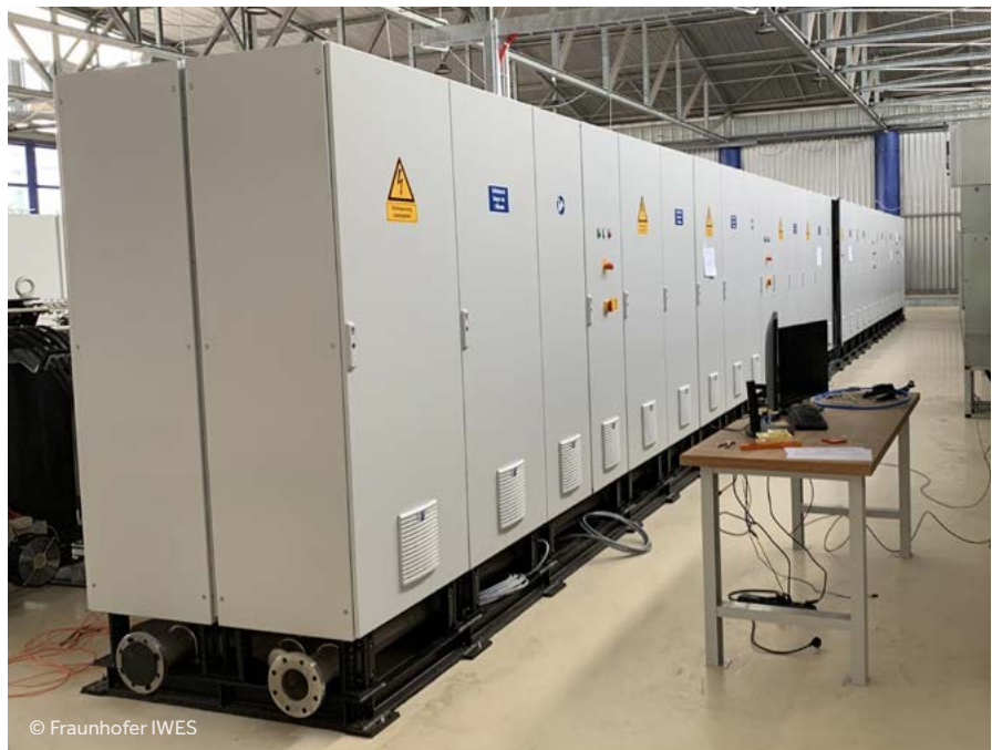
Converter cabinets of the PQ4Wind test bench containing a total of 20 megawatt installed converter power for emulation
