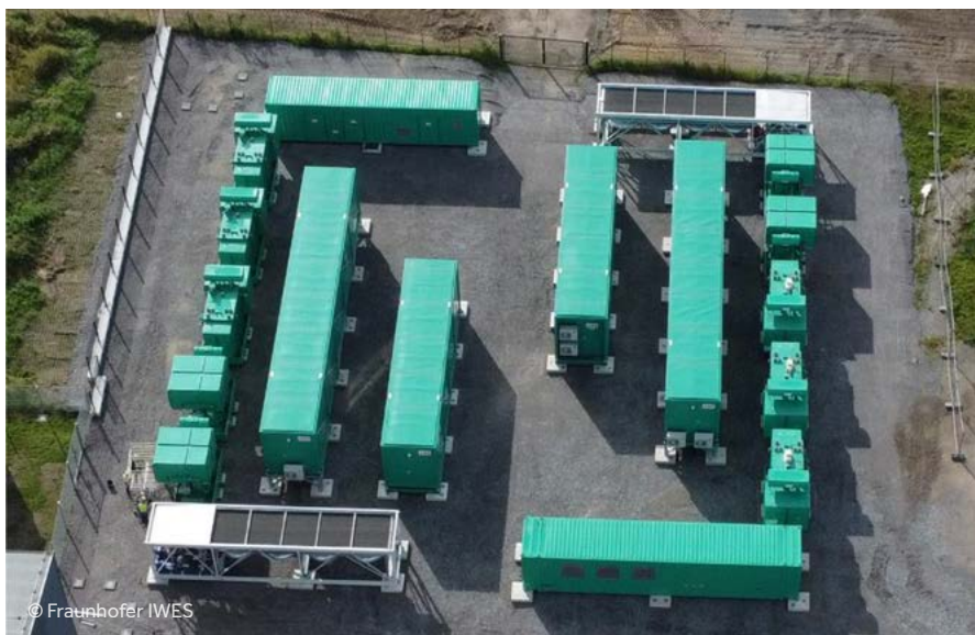
The 80 MVA mobile grid emulator. All components are housed in containers except the transformers
