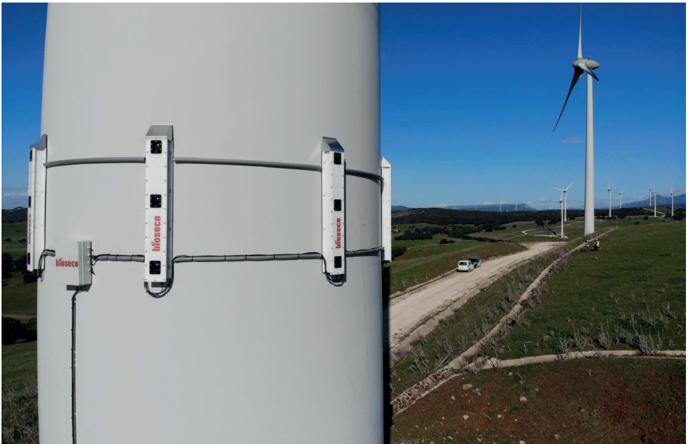
Bioseco systems installed in Spain during 2020
