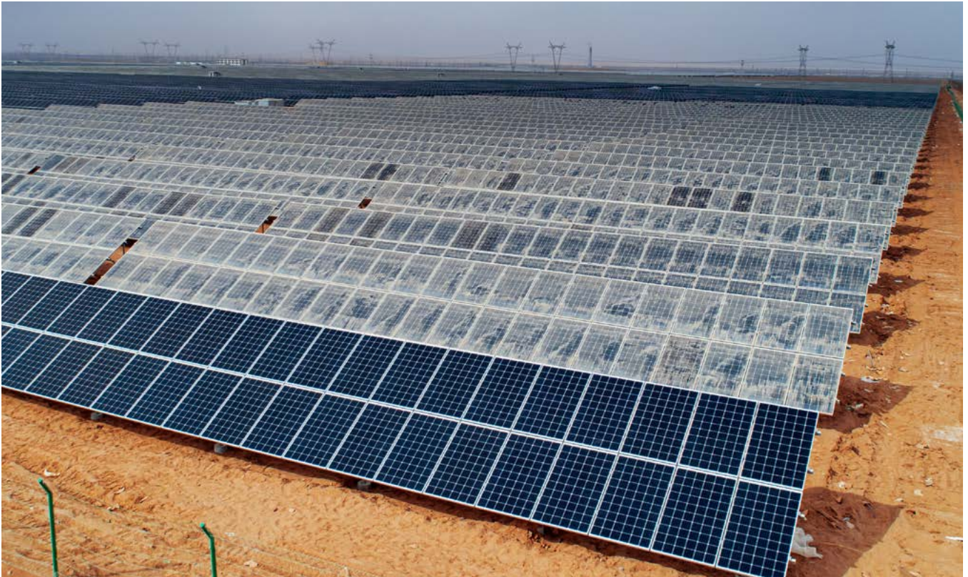
Soiled modules can significantly decrease power generation
