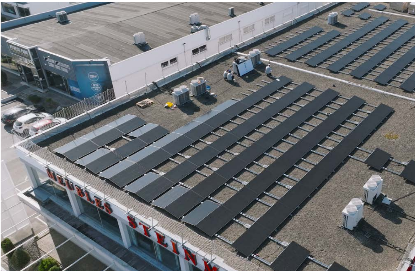
The QT2 on the roof of the Steinmetz furniture brand in Alsace, France
