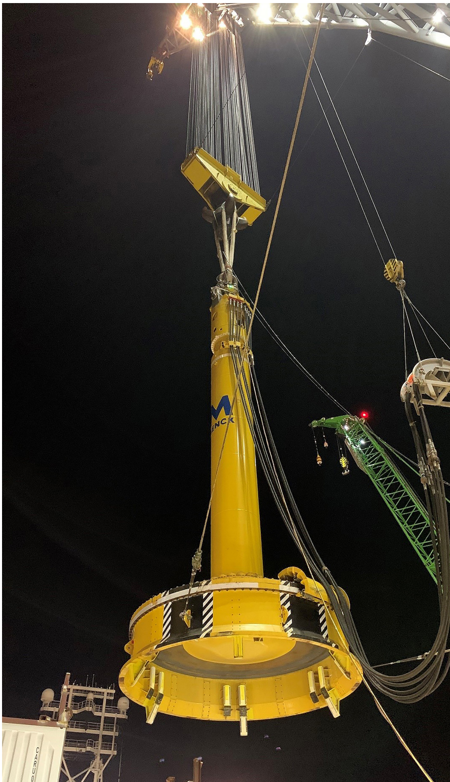
A MENCK hammer being used on Vattenfall's Hollandse Kust Zuid I-IV (HKZ) offshore wind farm project in the Netherlands
