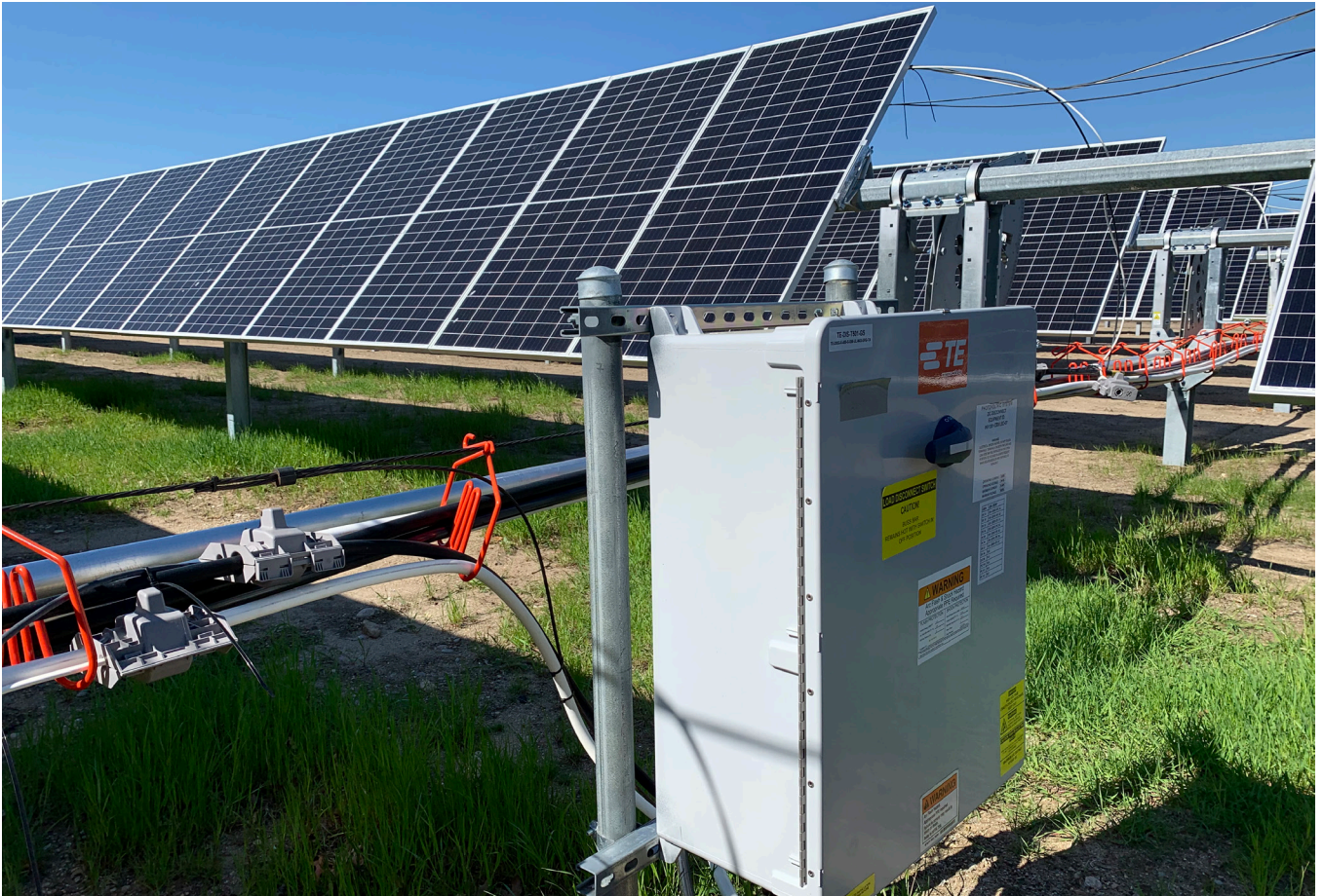
Solar IPCs and Disconnect Box
