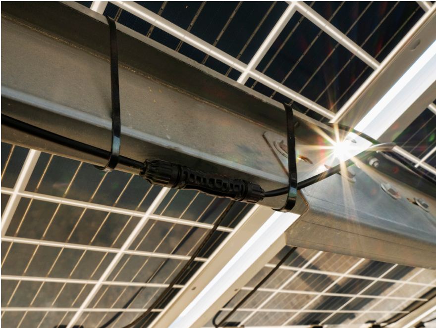
The DC wiring system with cable couplers, or eBOS, is the lifeline of a PV system
