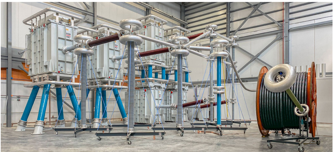
Resonant test system for very long cables
