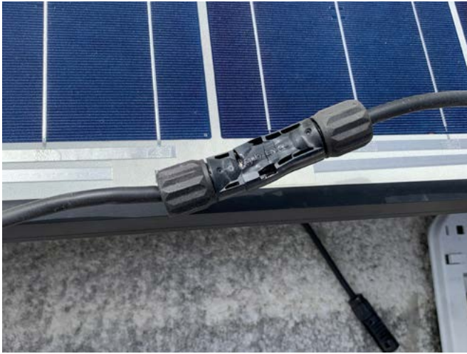
Figure 3: An example of a PV MC4 connector that has gone through stages of heating. If you don't test specifically for high resistance points in the string, you must inspect all connector sets to make sure that everything is on order. However, a visual inspection can require checking millions of connectors, so alternative testing principles are required to maintain the system ROI
