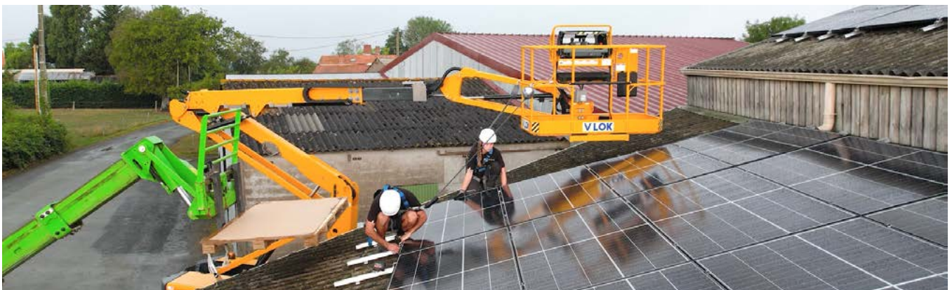
250 kWp agrivoltaics project carried out in Vendée, France
