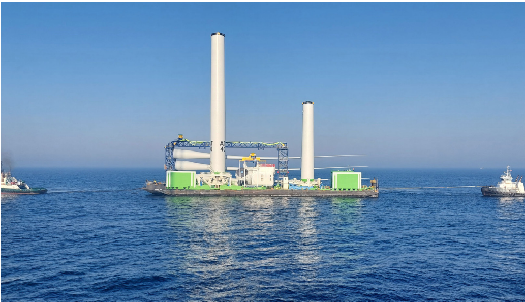
Photo: Installation Jack-Up lifting of a 50 meter tower section from the BM-Feeder.
