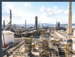
Digitalised Site Monitoring & Systems Auditing
