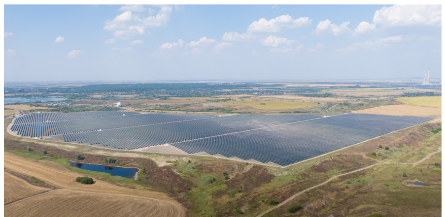
Producing 56MW of peak capacity, construction was recently completed on Bulgaria's first 1P L:TEC solar park
