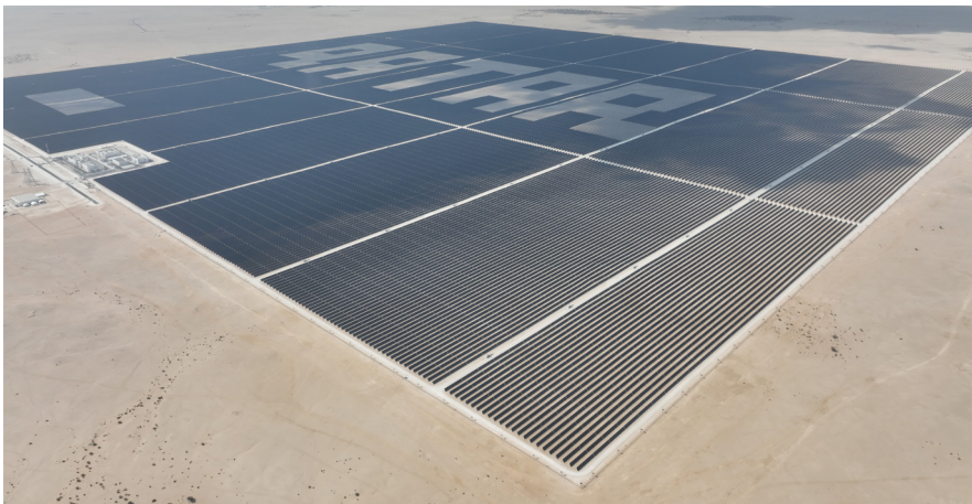
Generating 800MW of peak capacity, Ideematec has supported Qatar and its communities in constructing the largest 2P solar park in the world
