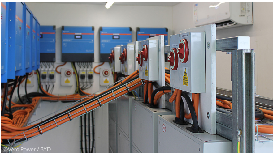
Energy management equipment and eight 15 kWh BYD Battery-Box LVL battery storage systems
