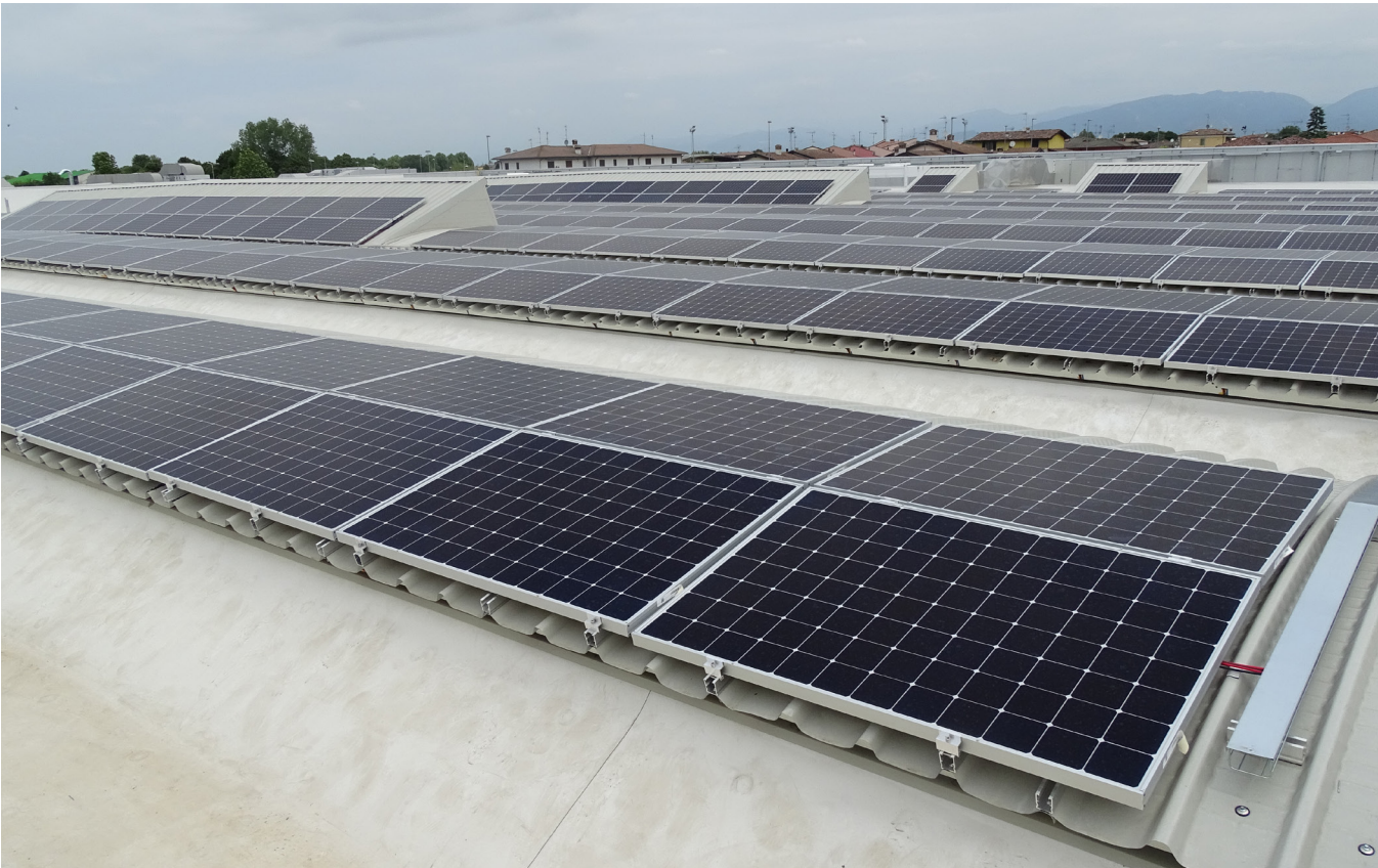
SolarEdge rooftop PV system at Italmark supermarket, Italy
