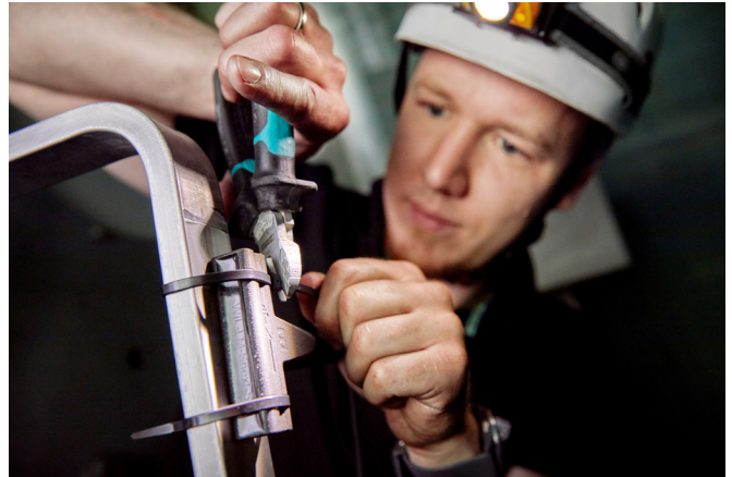
Figure 5: The sensor can be easily attached to the lightning arrester
