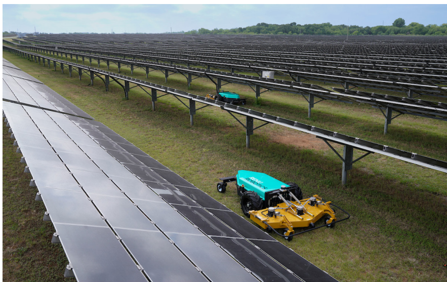
Two Renubots cutting grass on a utility-scale solar facility
