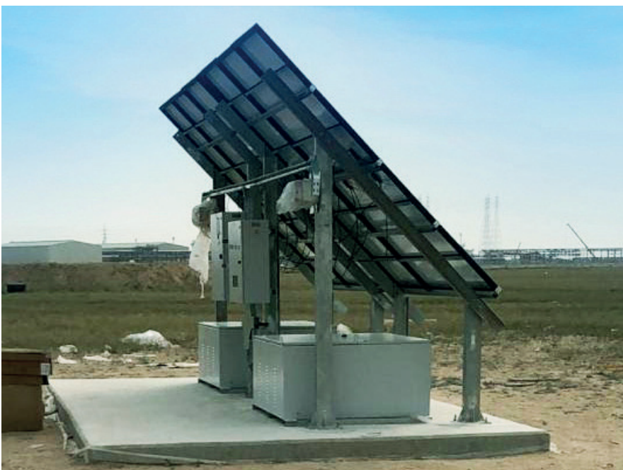
Solar electric array with Morningstar controllers powering oilfield lighting in the desert, for Kuwait Petroleum Corporation. Courtesy EcoSol Energy Systems
