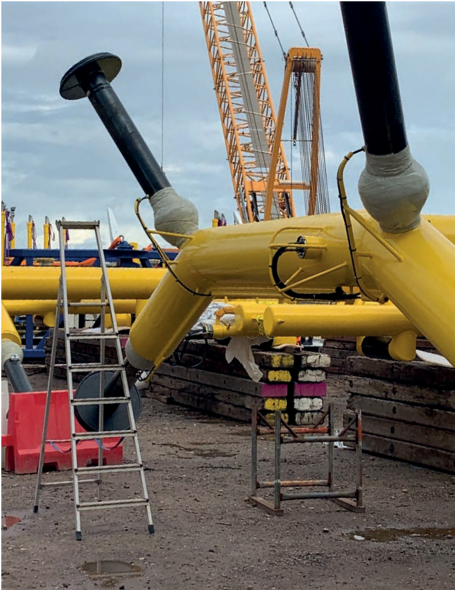
ICCP flanges close up
