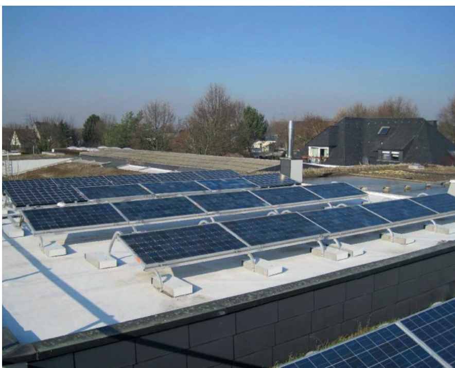
SolAround ISE Fraunhofer rooftop test installation - Geilenkirchen, Germany
