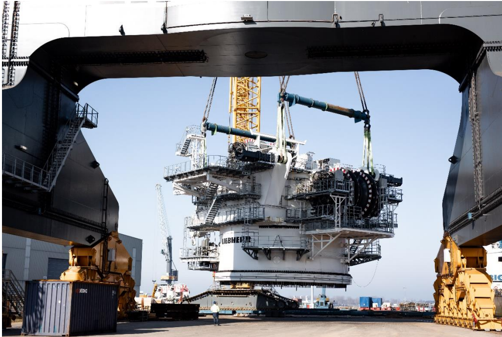
The slewing platform and the A-frame of the HLC 150000 have been lifted onto the BigLift Barentsz
