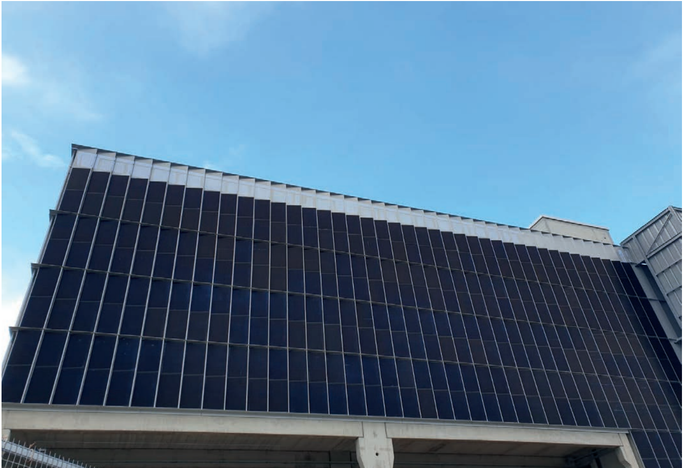
PV walls of a parking garage at the Helsinki-Vantaa Airport
