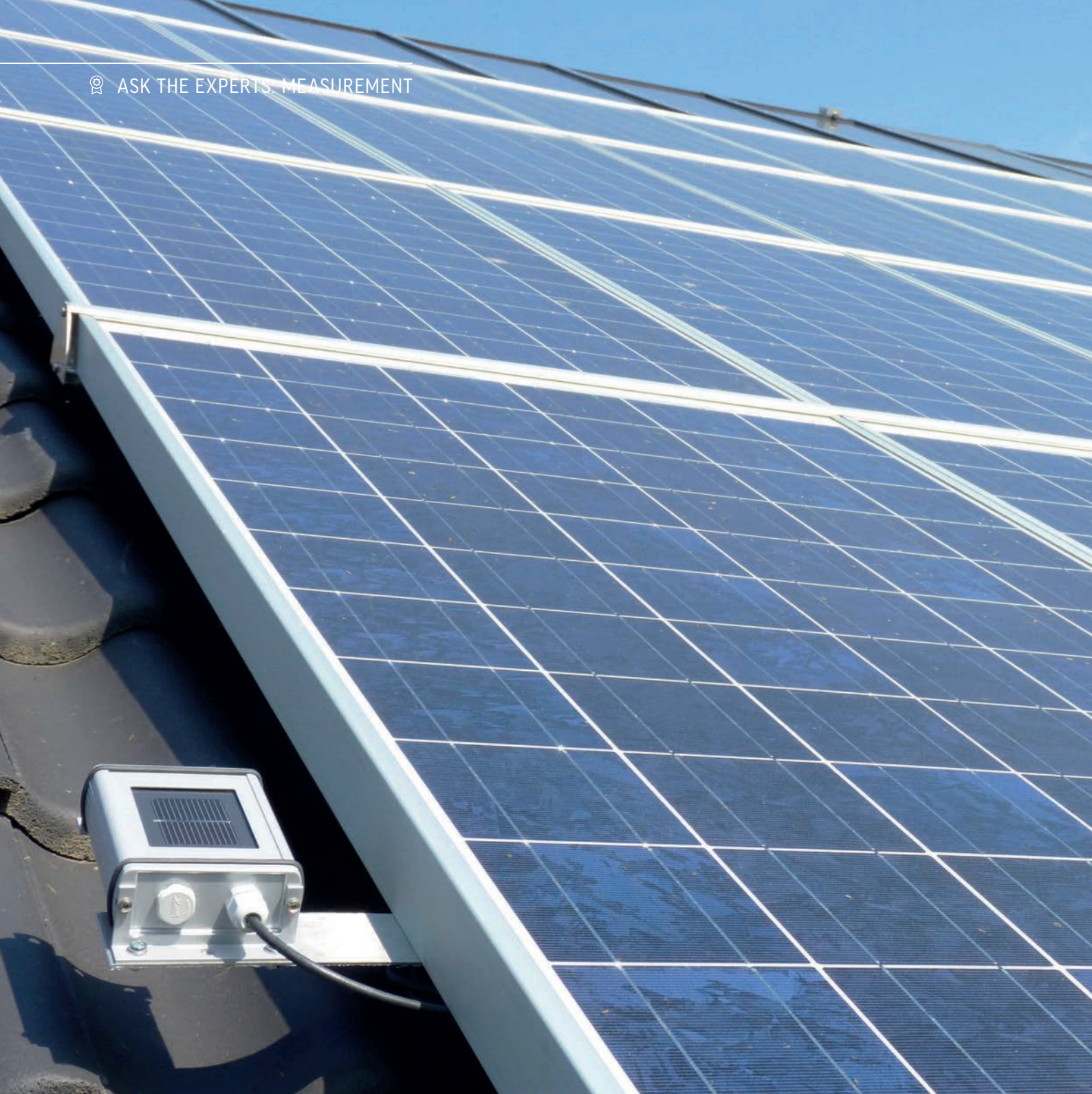
IMT Si sensor on a rooftop PV generator
