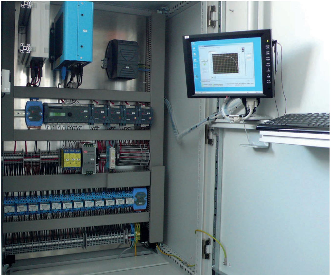
Automatic I-V curve measuring system for up to 12 PV modules (IMT)
