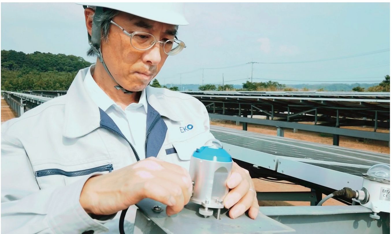
An EKO engineer installing a new MS-80S pyranometer at the EKO Inashiki solar park in Japan
