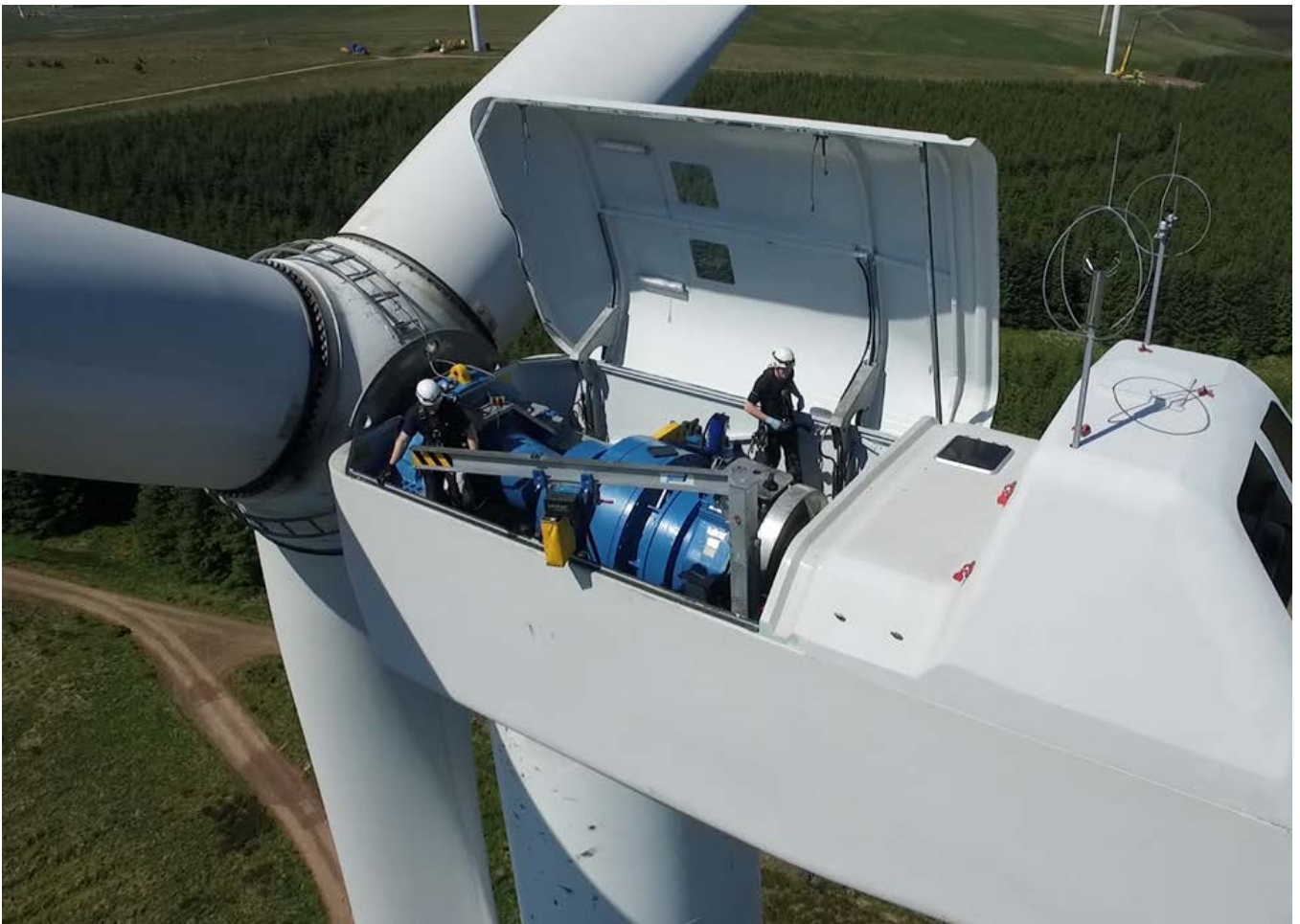
Natural Power's servicing team working with the APE team to deliver essential repairs
