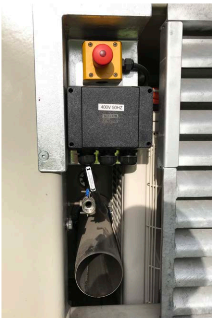
Connection point for potable water and sewage water at the containers
