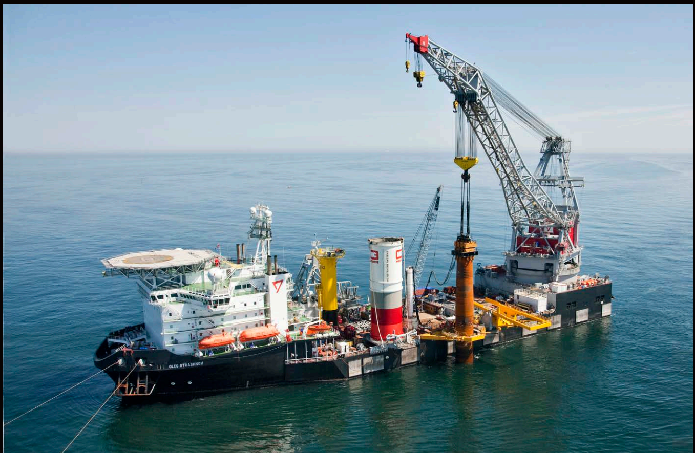
The first ever Mono Piles driven with a vibro hammer in offshore wind
