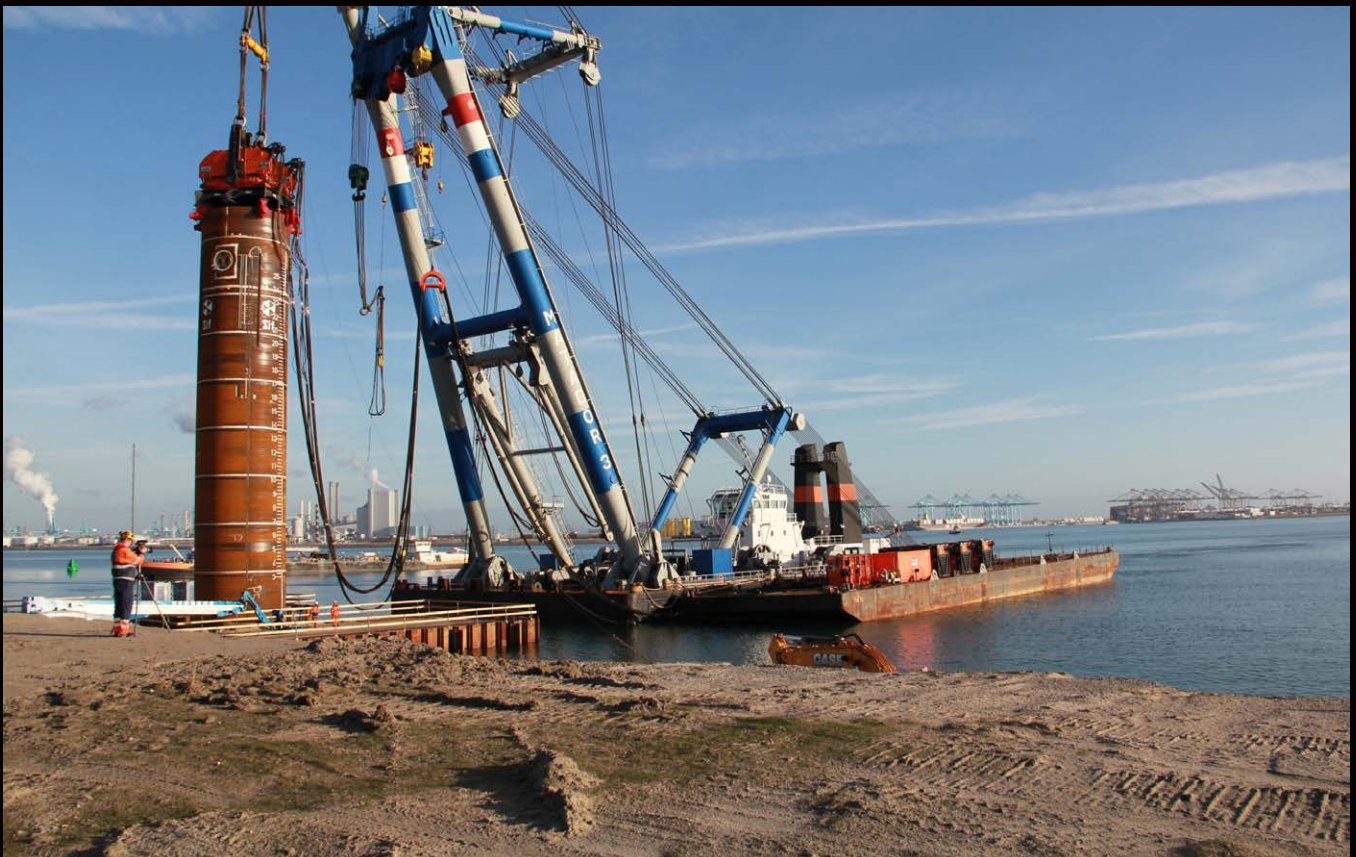
6.5m monopile at the Maasvlakte; 24-meter penetration in 15 minutes net driving time
