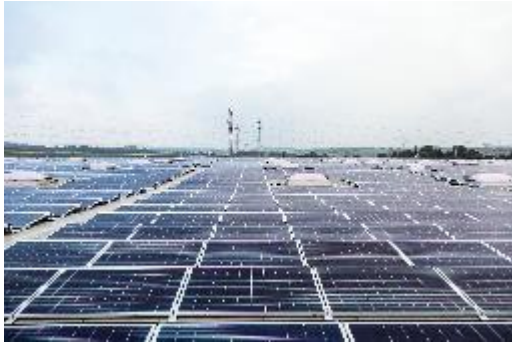
Image 3: Industrial buildings with their large flat roofs are often ideal sites for solar collectors.
