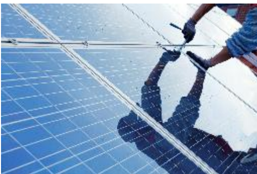
Image 2: Self-generated solar energy ensures greater independence from the public grid, reduces both energy costs and CO 2 emissions making it an important step towards greater sustainability.
