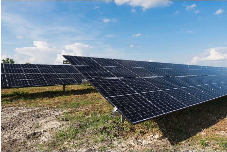
Image by Photon Energy: 3.5 MWp photovoltaic power plant Fertőd II in Fertőd, Hungary.
