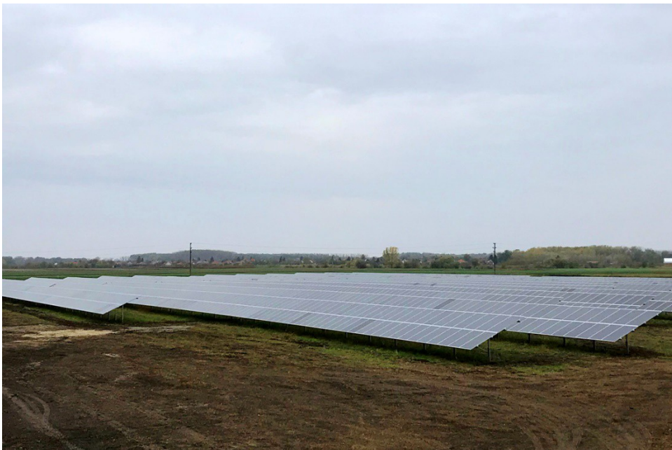
Image by Photon Energy: 1.4 MWp photovoltaic power plant in Kuszentmárton, Hungary.
