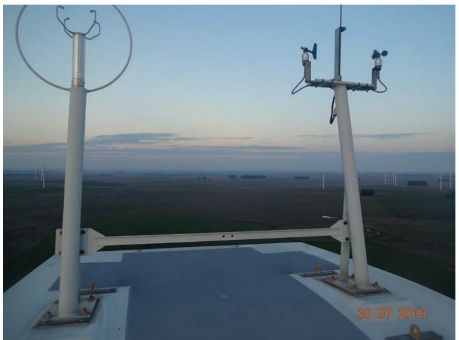
Anemometry looking out the back of the nacelle from the roof
