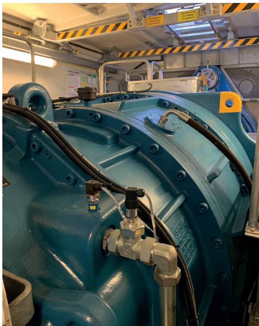
Gearbox from the back of the turbine facing the rotor
