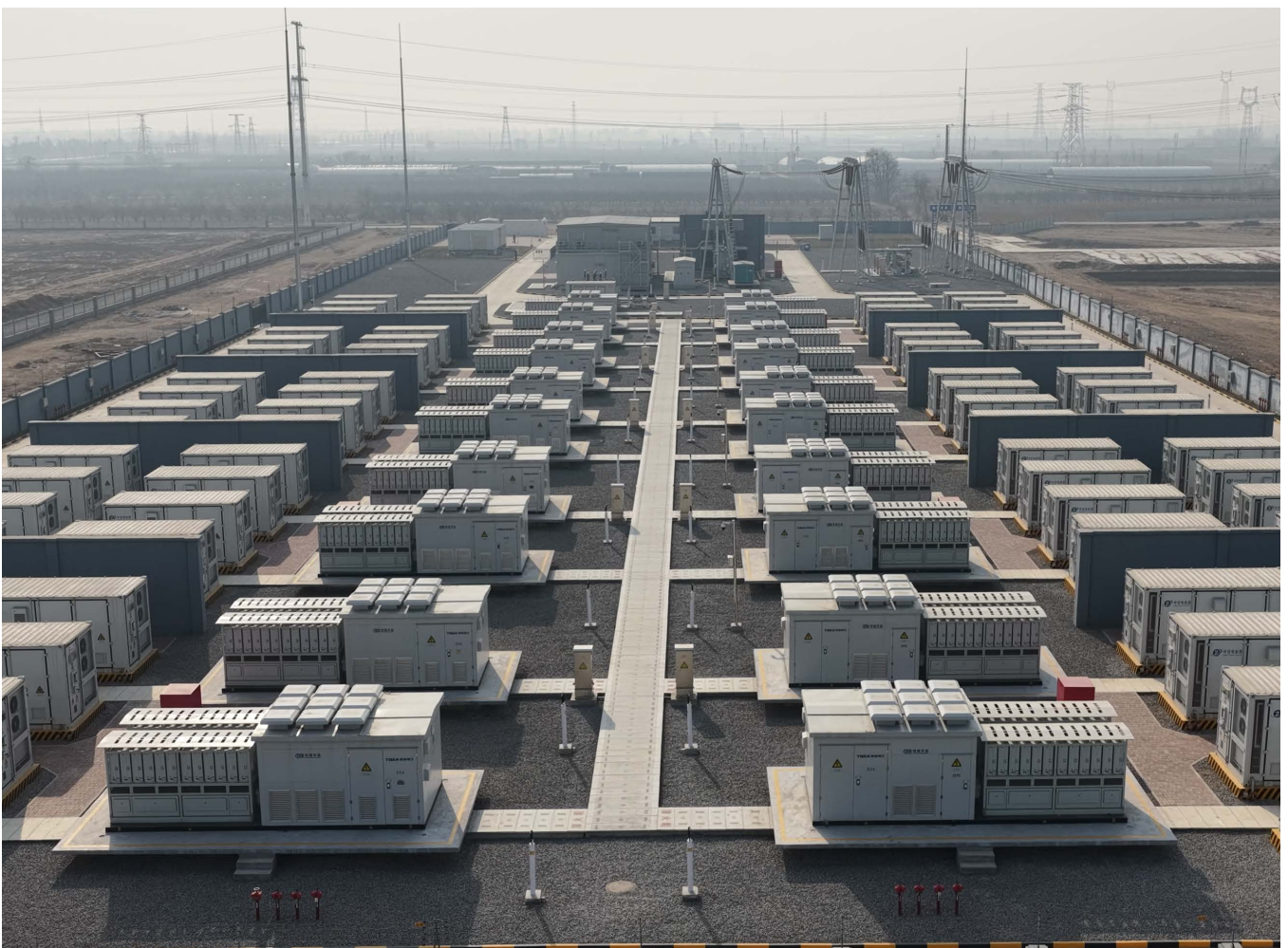
100 MW APStorage project Longteng Factory in Shenzhou, Hebei Province, China
